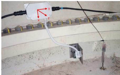
LVDTs at the tower base
